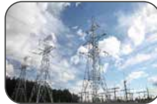
Power line stations
